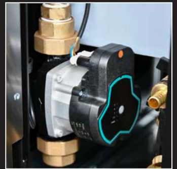
Circuit pump of heating
